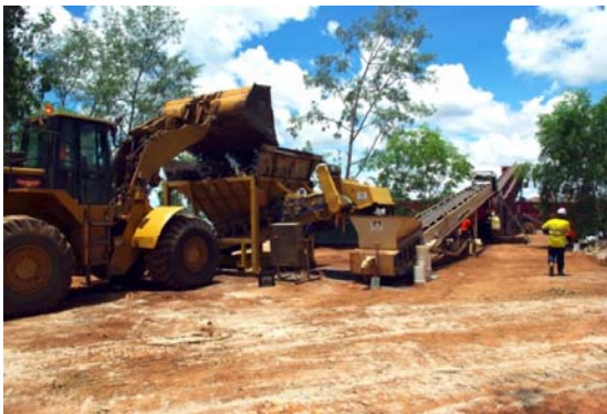
Front end loader feeding concentrate onto conveying system
