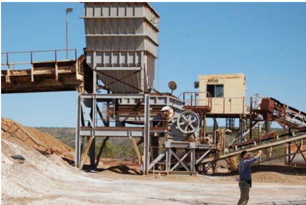
ROM Bin & Crusher
